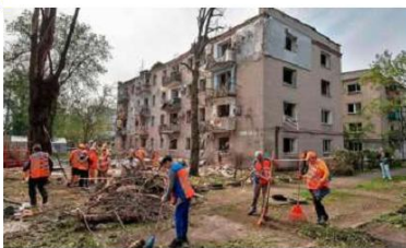
Picking up the pieces: Municipal workers clean debris following an air attack in Dnipro on Monday. AFP
